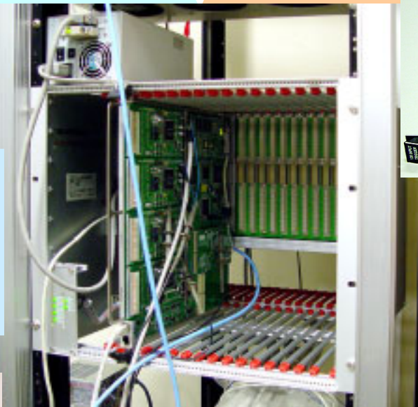
KEK-VME crate VME crate with extended power supply
